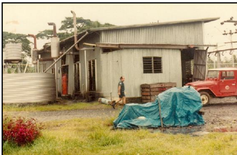
Kimbe diesel power generators
