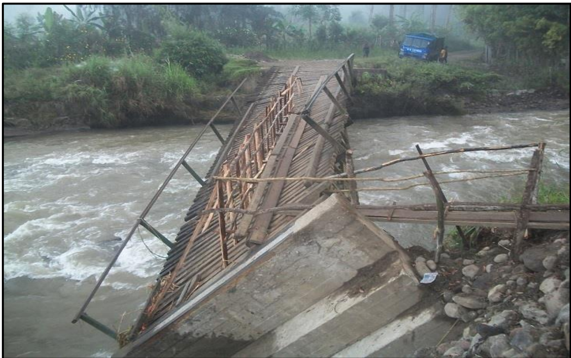
Illustration 10.2.4a: Wapenamanda affected by floods and landslides. Topak Bridge affected by floods.
