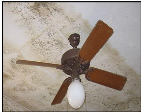
Mildew (mold growth) on the ceiling and walls
