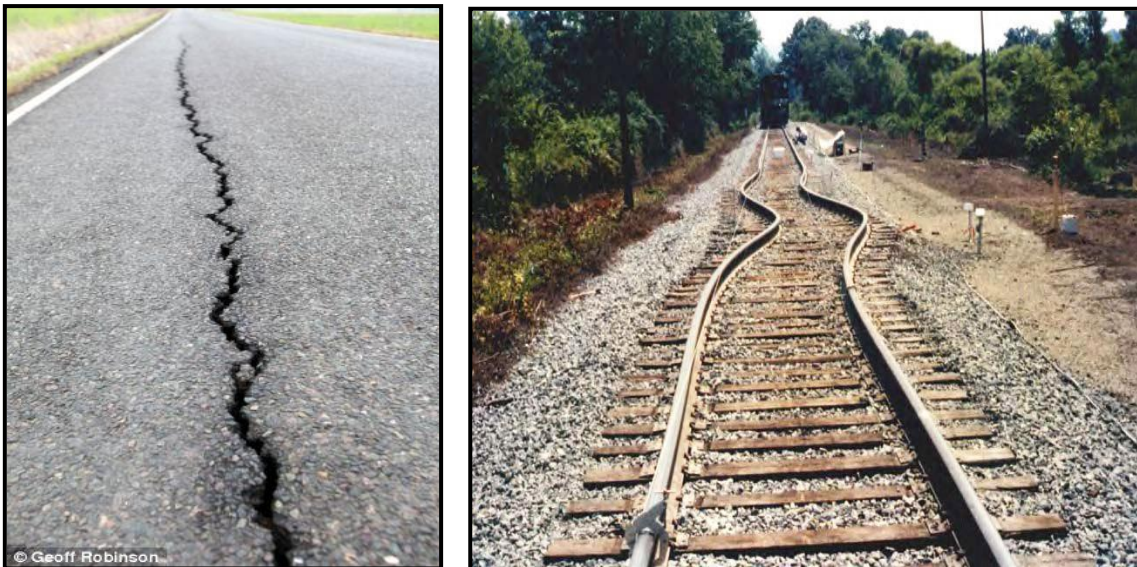
Figure 5 Effects of thermal expansion on roads (left) and railway tracks (right)
